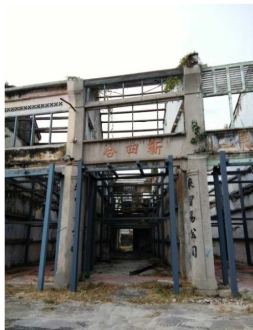
Figure 5 The current condition of the exterior (left) and interior (right) of one of the shop houses at Sia Boey. (January 2017)
